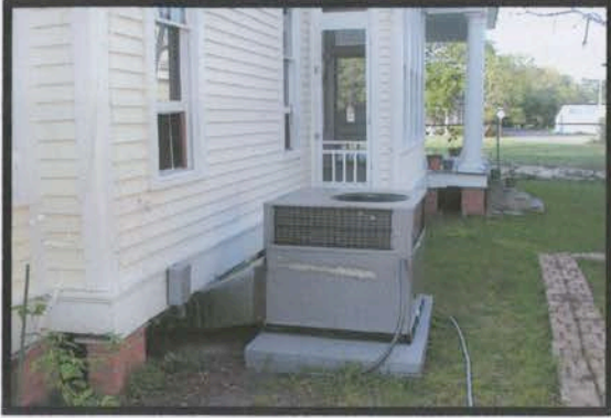
New central air and heating unit can be seen on the East side of the house.
