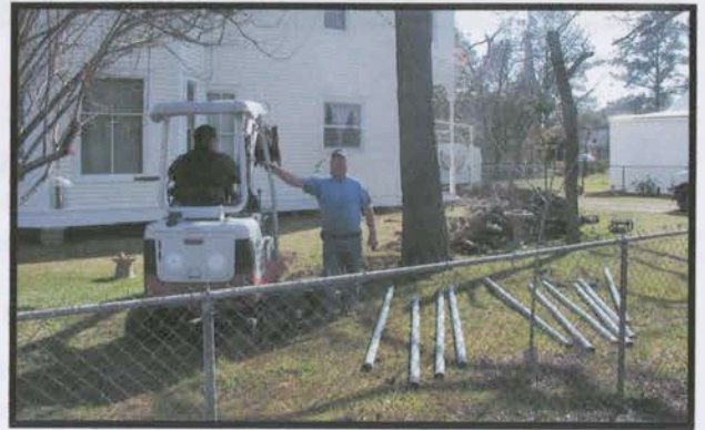
Neal Shelton and son Raymond install underground electrical wiring at Hewes House in January 2006.
