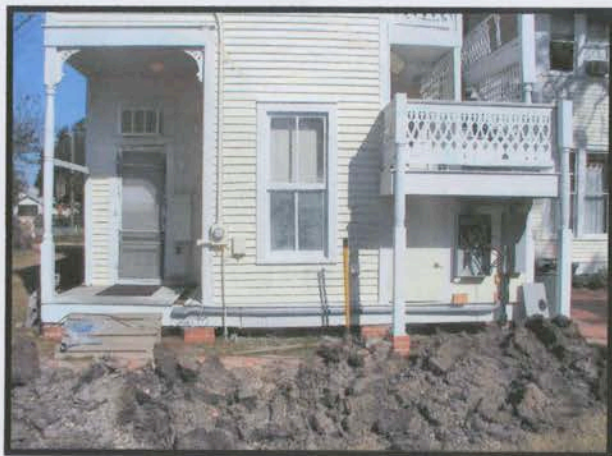
Rear picture of Hewes House shows new electrical panels and underground work in progress.
